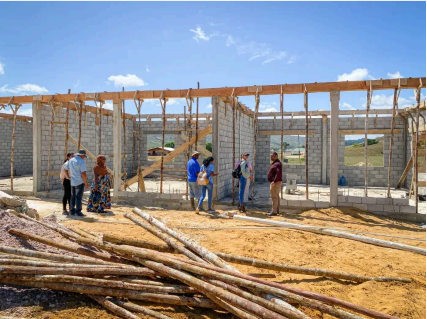
Construction ongoing at the Monkey Mountain Secondary School in Region 8 (Photo: MoE/December 2024)
